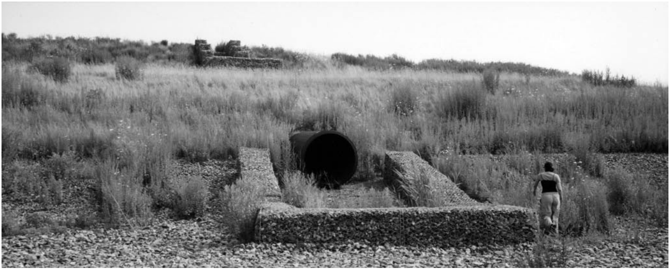
A still photo of the Fresh Kills landfill drainage system taken from a six-channel video installation featuring the many people involved in envisioning the future of the country's largest land fill. Photo courtesy of Ronald Feldman Fine Arts
